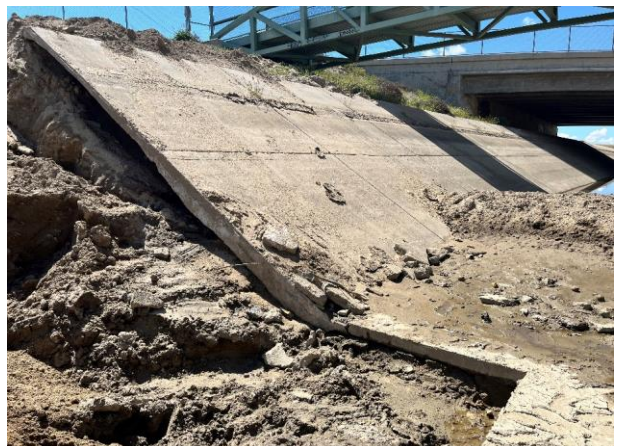
Existing concrete liner damage to be repaired.
